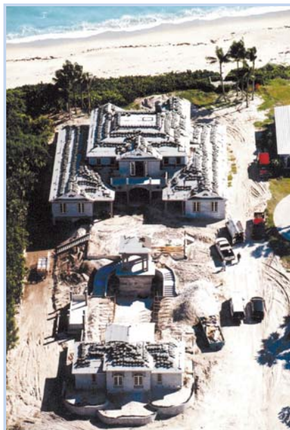
Mid-point of project shows all interior and exterior walls complete and roof ready for tiling.
