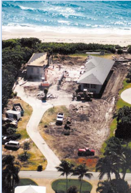
Surgically precise demolition was necessary to prepare old foundation for new construction.
